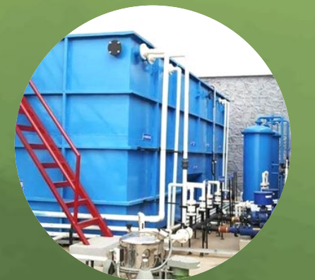
Sewage Treatment Plant (STP)
